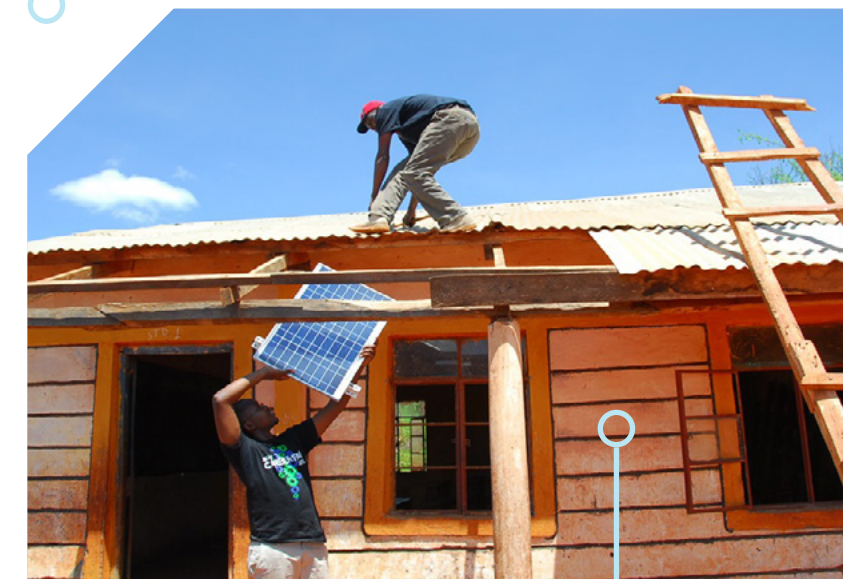
IEEE's Kenya student branch installs solar panels at the isolated Kasiluni Primary School, the only institution of its kind within a 25-kilometer radius. The school serves 600 pupils in six grade levels.
